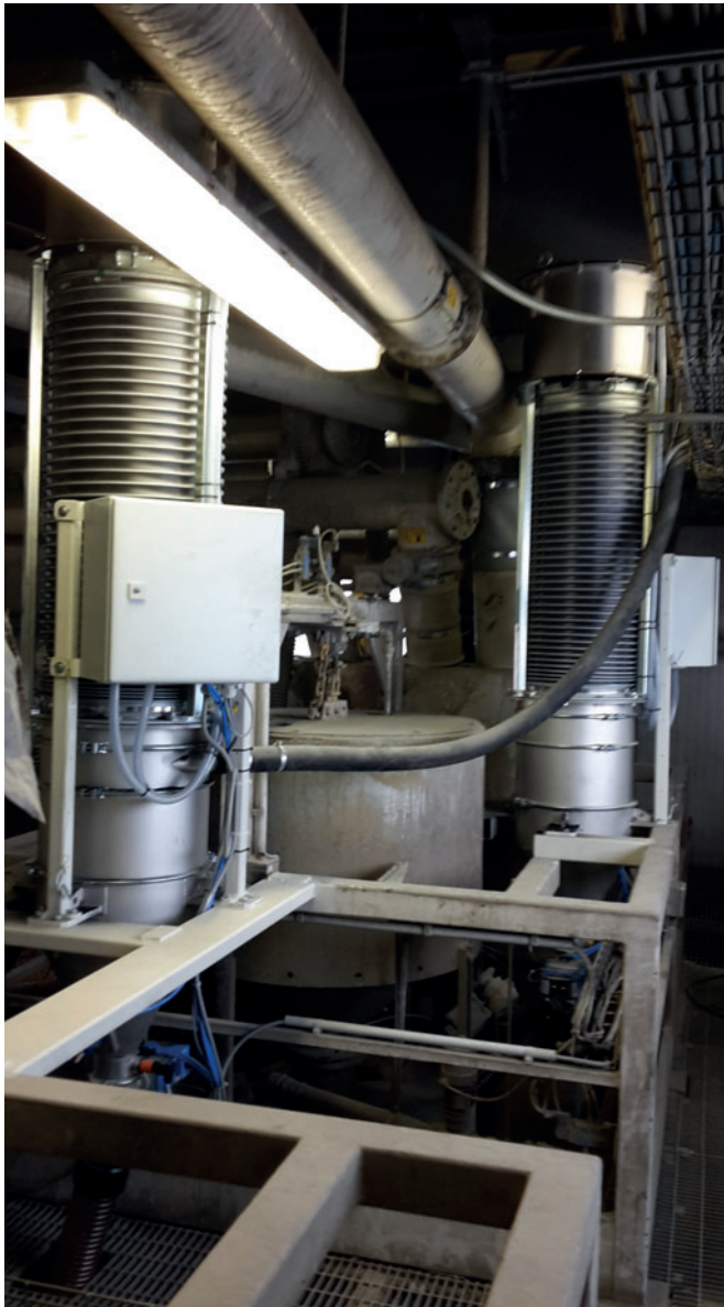
Filter cyclones above the concrete mixers
