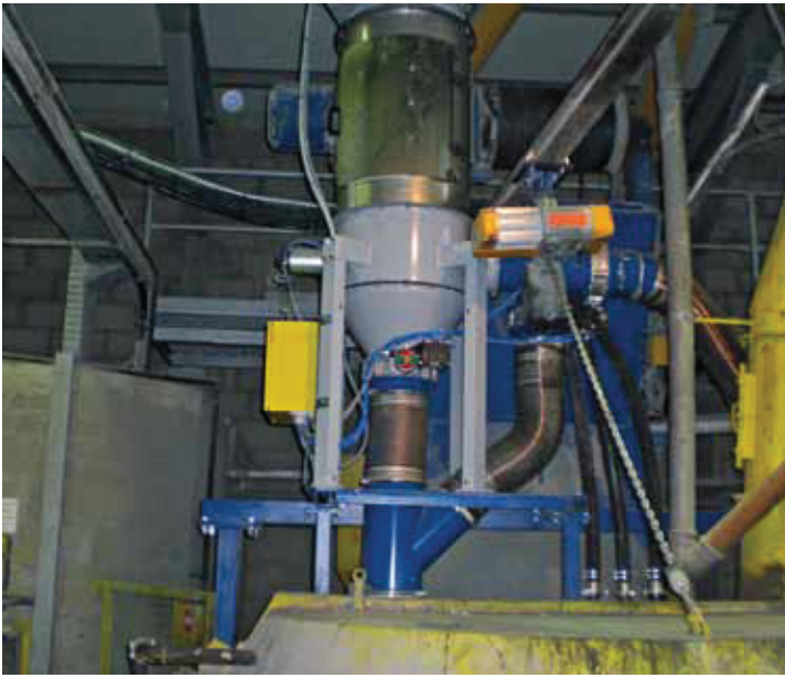
A motor-powered suction system was installed to prevent dust from being emitted from the mixers
